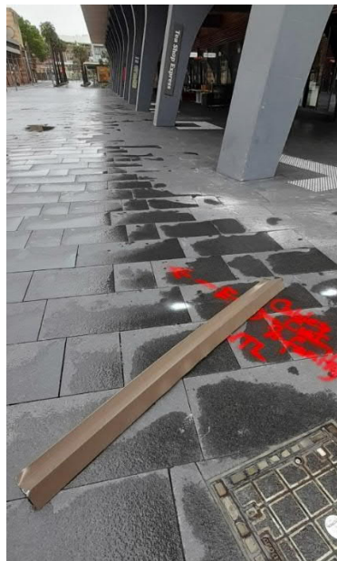
Photo: fallen Façade flashing
